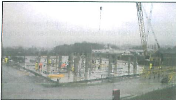
Photos showing the site offices / welfare and the precast columns being erected
